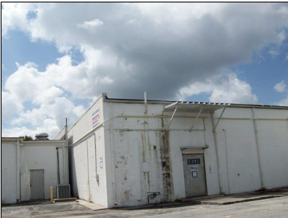
Deteriorated commercial structure with compromised external surface and aging utilities.
