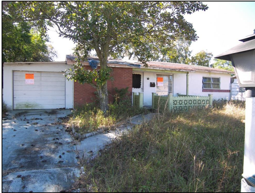
Deteriorated/unsafe structure with significant roof damage.
