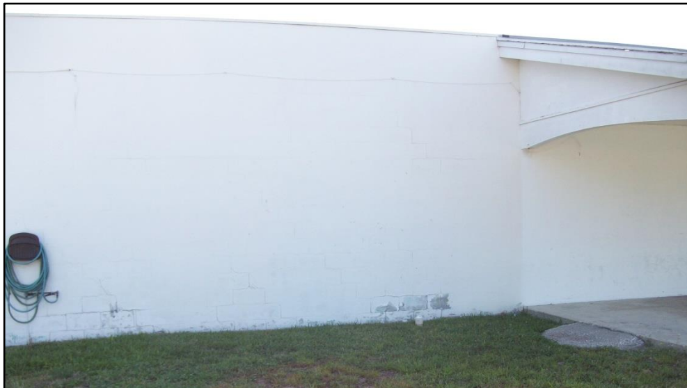
Deteriorated commercial structure with significant structural settling.
