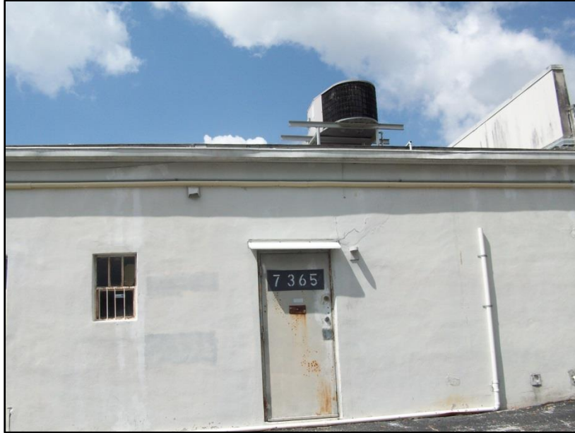
Deteriorated commercial structure with significant deterioration visible on doors and windows, and, aging climate control system on roof.
