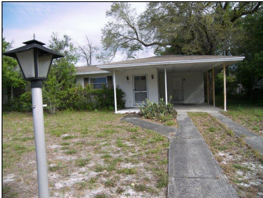
Signs of structural deterioration visible on doors and supports.
