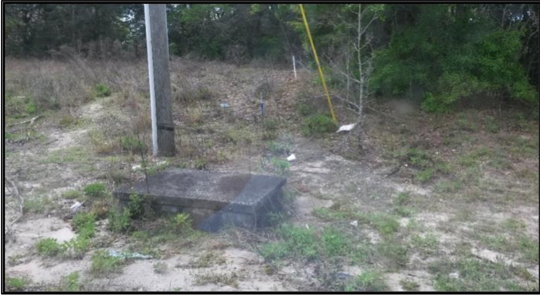
Figure 27: Unsafe and Inadequate Drainage Facilities
