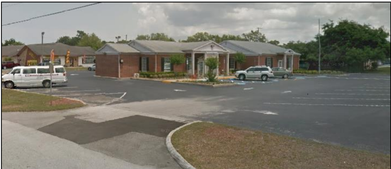
Figure 8: Fragmented Pavement Repairs
