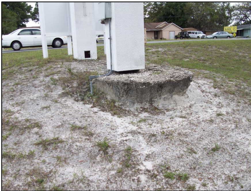
Large deteriorated and aging commercial sign structure with significant foundational compromise.
