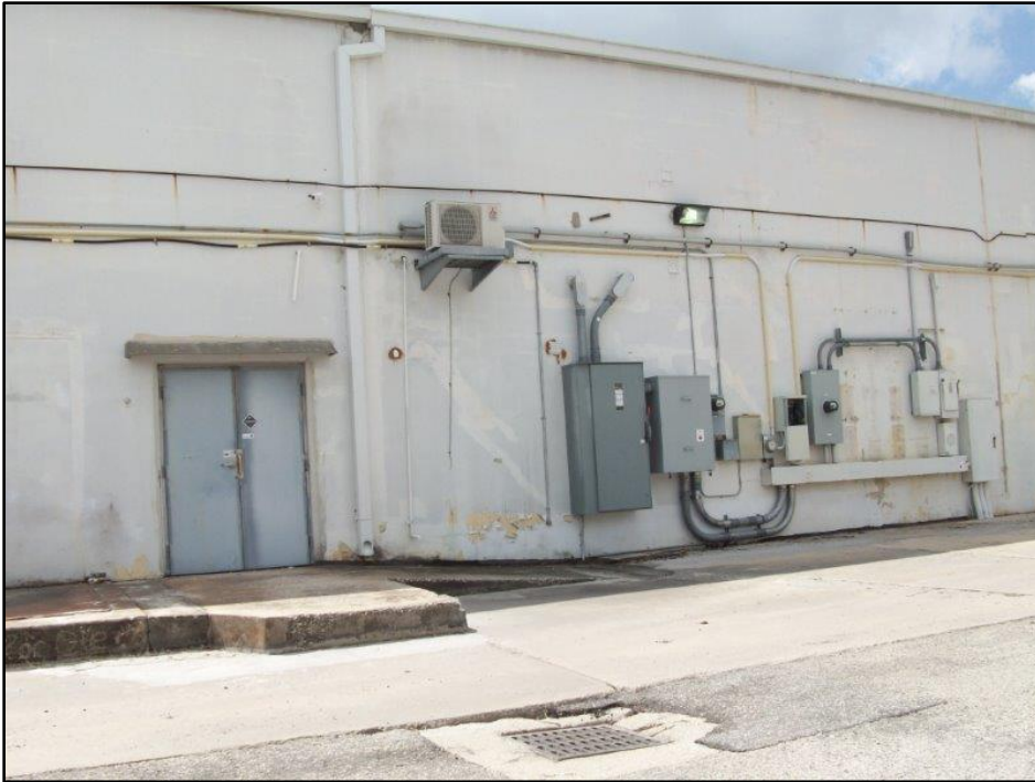
Deteriorated commercial structure with abandoned and aging utility infrastructure.
