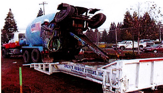
Commercial portable metal washout with truck ramp
