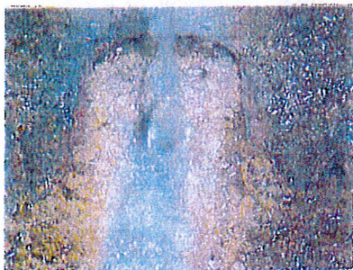
Figure 1: Sewer line filled with restaurant grease.
