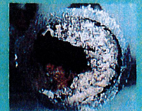
Clogged Pipe Caused by improper grease disposal
