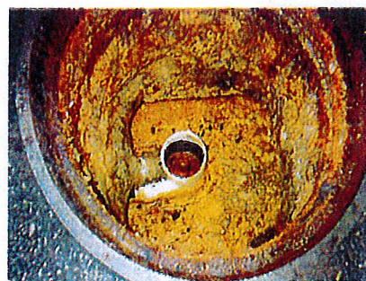
Figure 4: Clogged pipe due to FOG.
