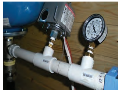
Water Pressure Meter
