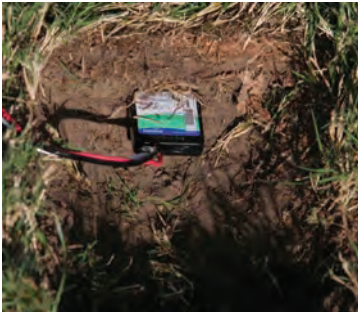
Soil Moisture Sensor Installed
