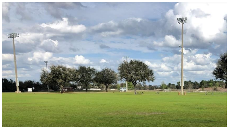
Figure 10: Anderson Snow Soccer Field Lighting
