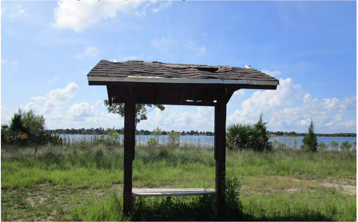
PHOTO 9: Existing, dilapidated pedestrian resting bench with roof, in Weeki Wachee Preserve.
