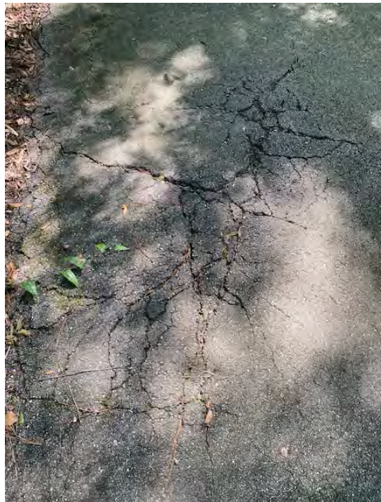
Root heave - typical, right side
