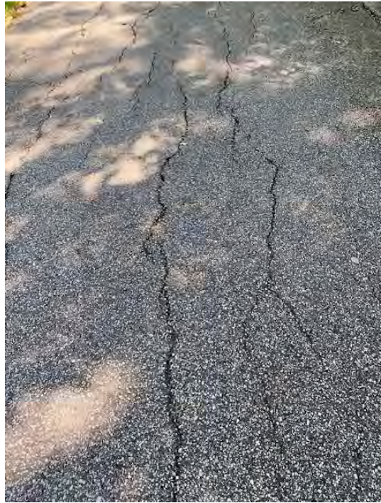
Longitudinal cracking - typical
