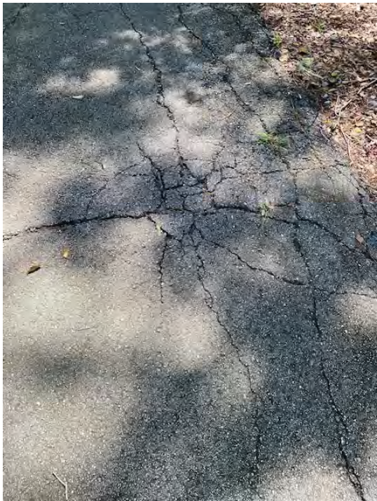
Root heave – typical, left side
